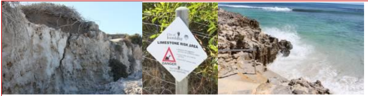
Figure 44: Limestone Cliff Risks and Management Issues
