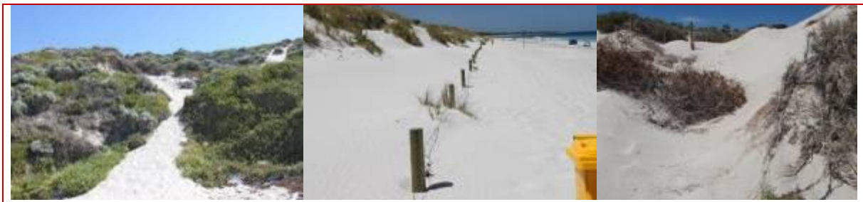
Figure 34: Erosion Examples within the Coastal Foreshore Reserve
