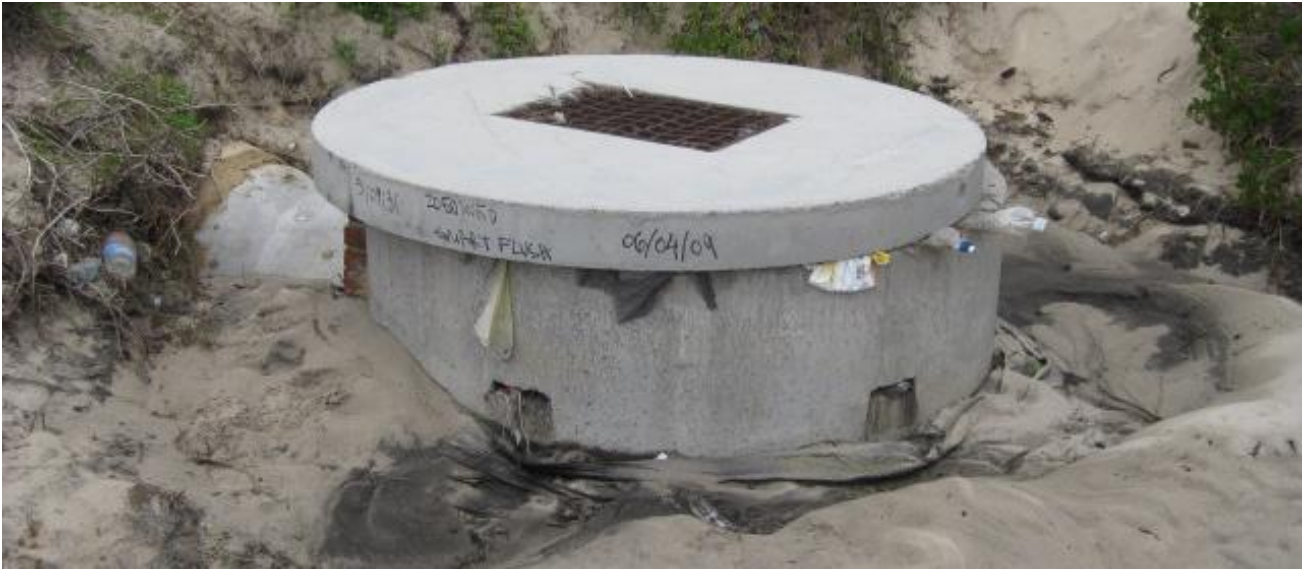
Figure 25: Drain lid movement caused by storm surge and expelled rubbish (Photo © M. Norman)
