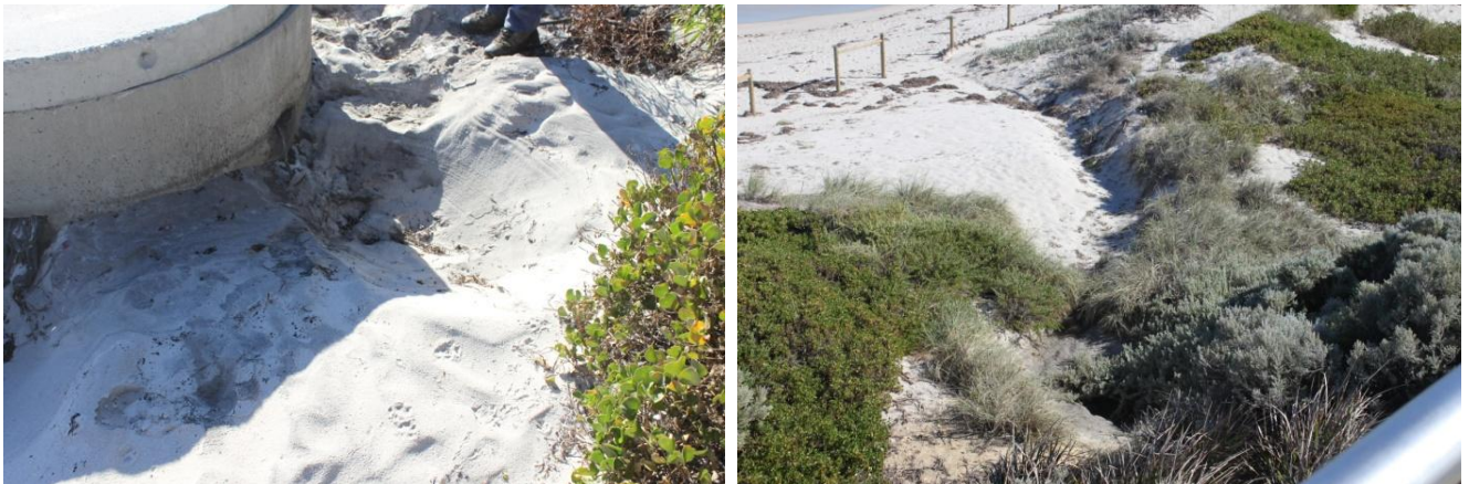
Figure 6: Erosion around stormwater drains creating gullies towards the beach within the site
