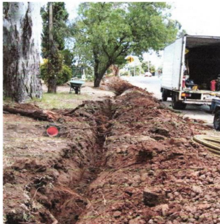
Photo: Showing tree root damage from service trenching within the TPZ.
